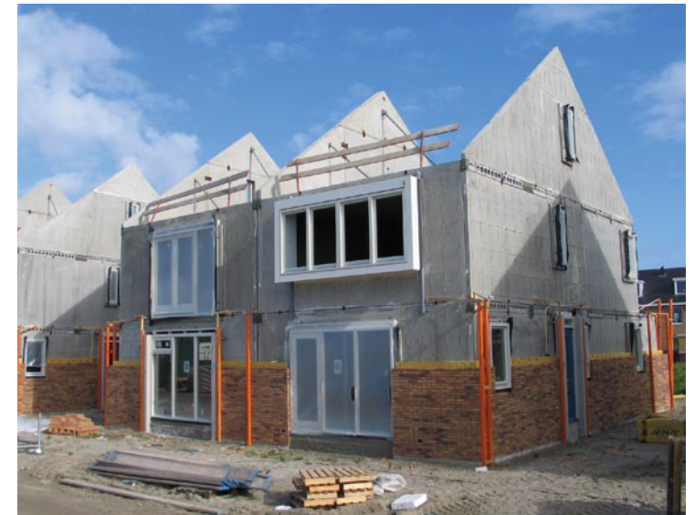
Lightweight concrete blocks are widely used in foundations and external walls for small houses because they are easy to lie and easy to work with. Courtesy of BFBN.
